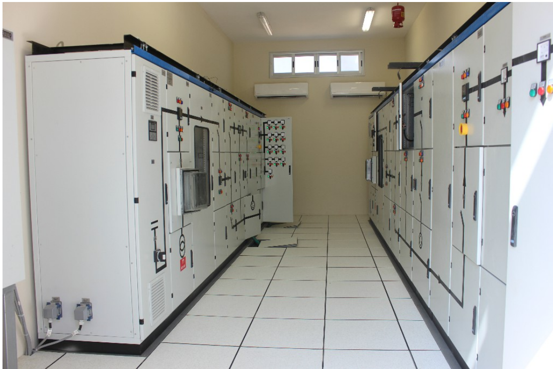
Installed Electrical Panels up to August 2019
