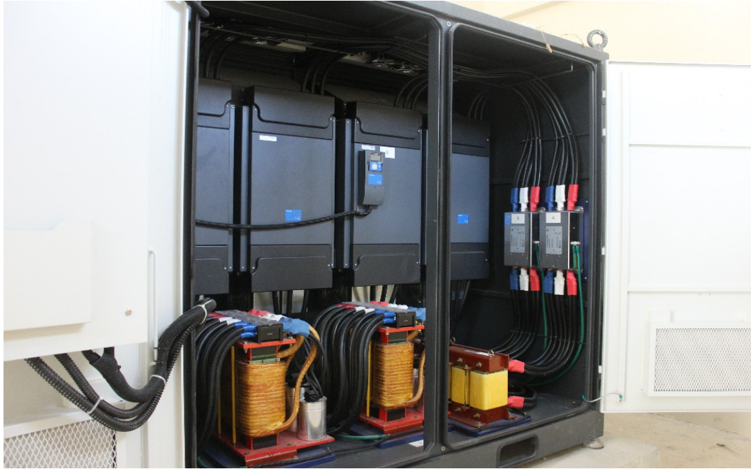
Installed Electrical Panels up to August 2019
