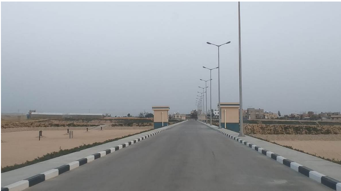
Accomplished Works of the Infiltration Basins up to Handing Over in April 2019
