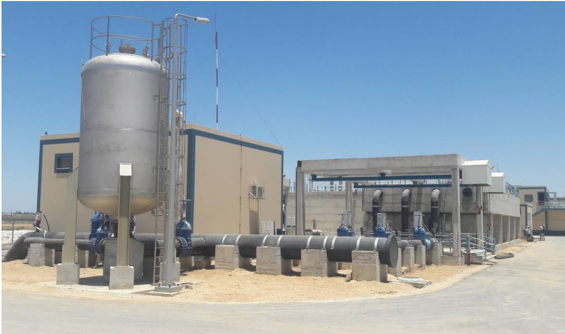
Installed Manifold and Surge Tank for Effluent Pumping Station up to August 2019
