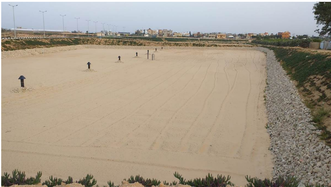
Accomplished Works of the Infiltration Basins up to Handing Over in April 2019
